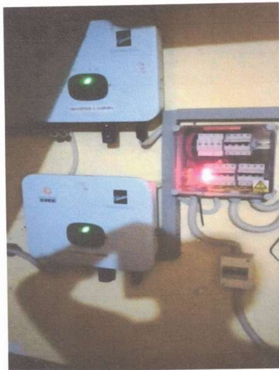
Solar panel photo and inverters
